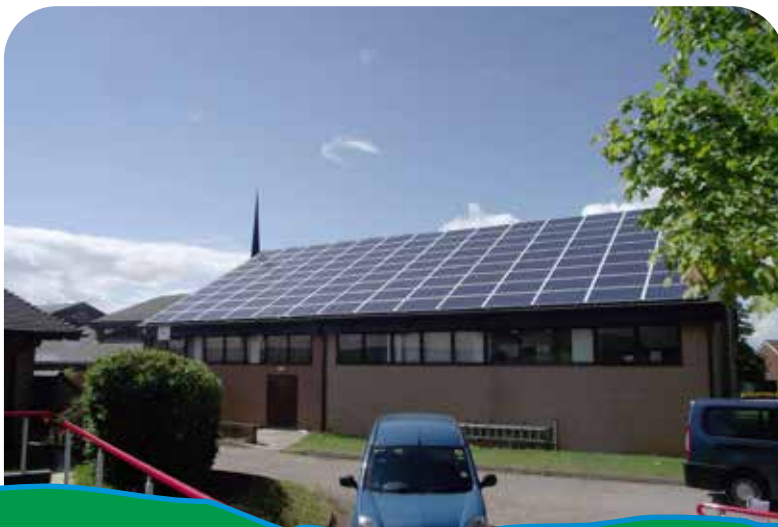
Solar power at Christ Church Bayston Hill
